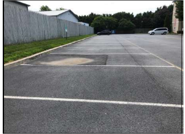
Asphalt parking lot - areas of sinking
