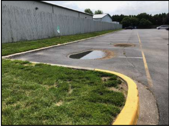
Asphalt parking lot - areas of sinking
