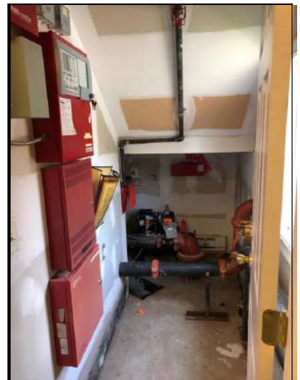
Typical fire suppression equipment
